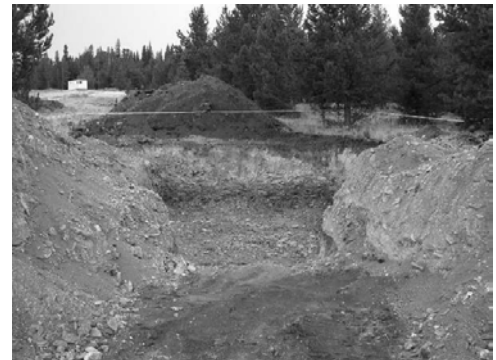
Currently all that is seen is the empty hole near the Dubois Fire substation on Union Pass.
